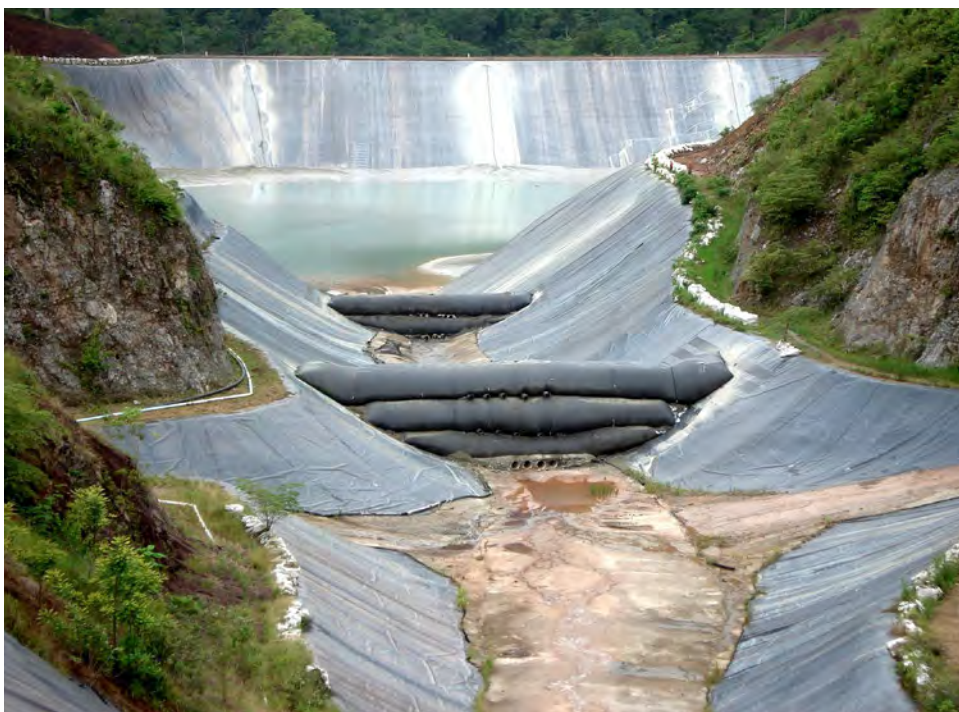
Geo-tube Dam's In Honduras. TenCate's Geotubes® have been deployed for "the construction of two dams in a river bed near a storage lagoon for mine tailings slurry in Honduras. The technology ensures storage, dewatering and filtering of polluted ground." 9
