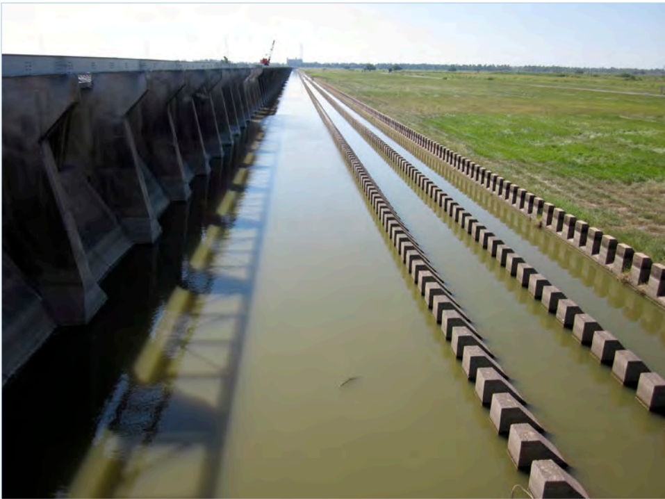
The articulated concrete surface at the base of the Bonnet Carre Spillway flood bays; image from the US Army Corps of Engineers.
